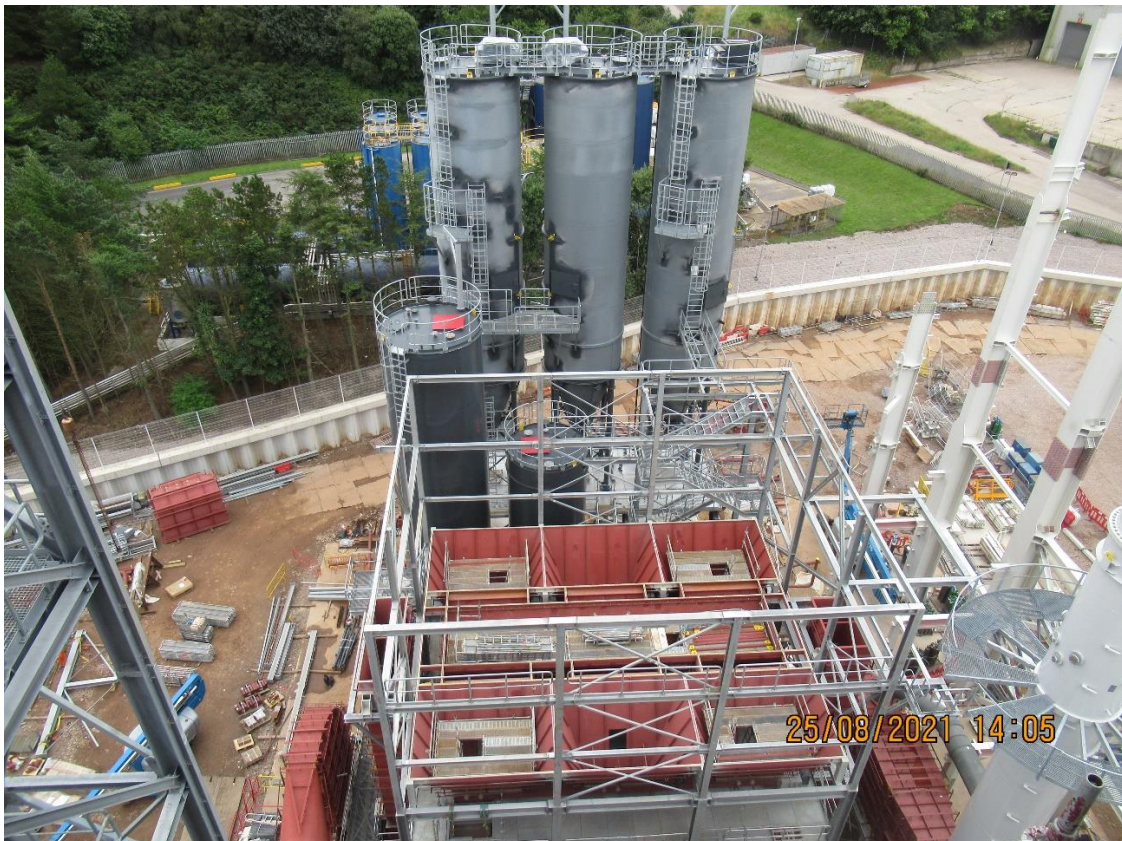
Flue Gas Treatment Area
