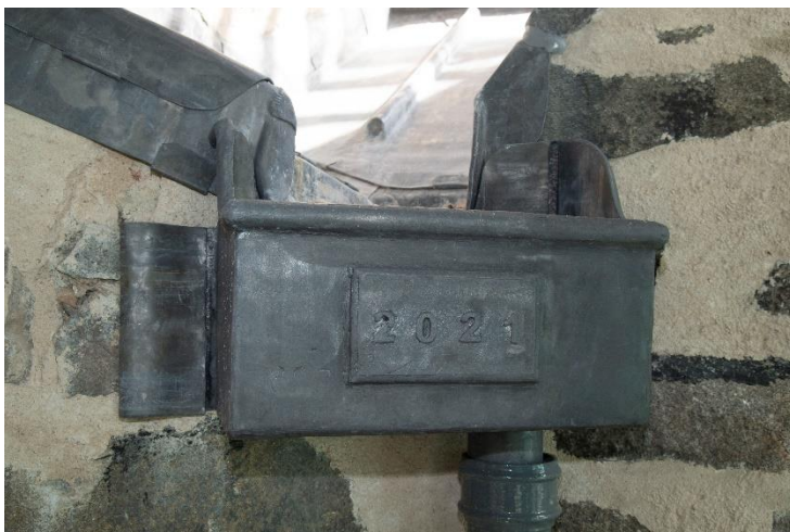
Handmade lead rainwater hopper
